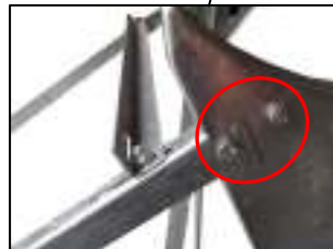
The collector's Π supporters are adapted to the tank's supporters with two bolts and nuts.
